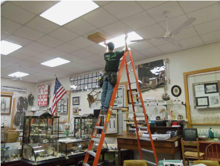
The new lighting being installed throughout the museum in Laporte by AEGIS Resource Management by David Clark & Kevin Coles (pictured) on 1/12/2016. This shot being taken in the Pauline Holcombe wing of the main building.
